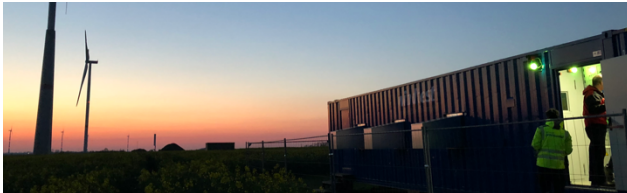
Figure 3: The first medium voltage auto transformer based test device owned by an independent test laboratory. Windtest Grevenbroich uses this frequently for many different power generation units.
