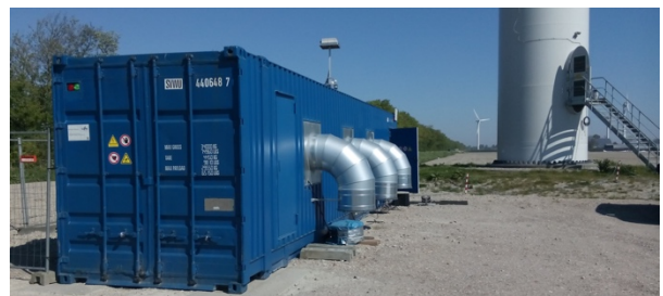
Figure 1: First auto transformer based test devices installed close to multi megawatt wind turbine.
